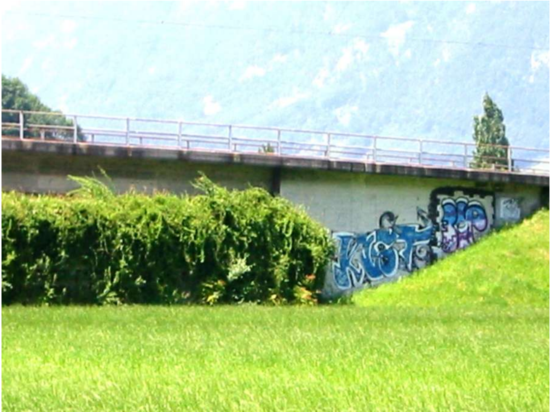
A Sound Wall along the Highway A2 near Lucerne, Switzerland: Any Graffiti on the Evergreen sound wall on the left? NO! only on the bridge abutment of course!
