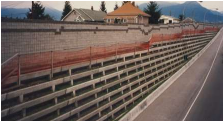
Cassiar Connector, Vancouver, BC – numerous walls
