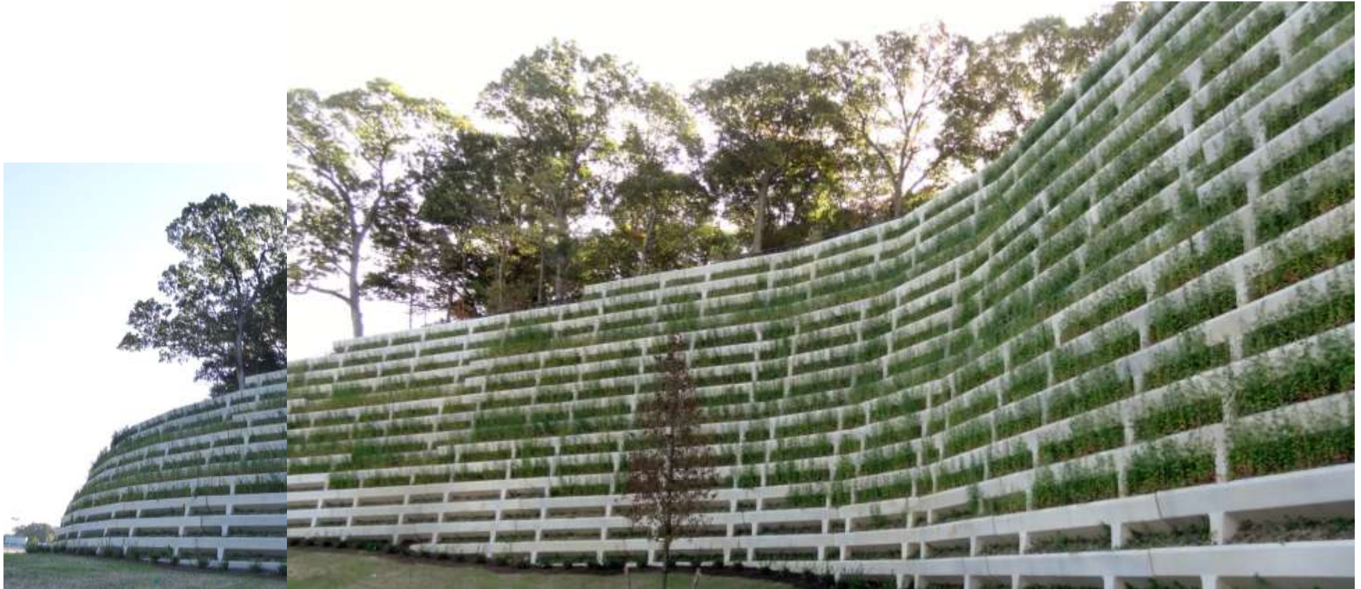
Swing Around Retaining Wall for Target Shopping Center in Huntington, Long Island, NY,
